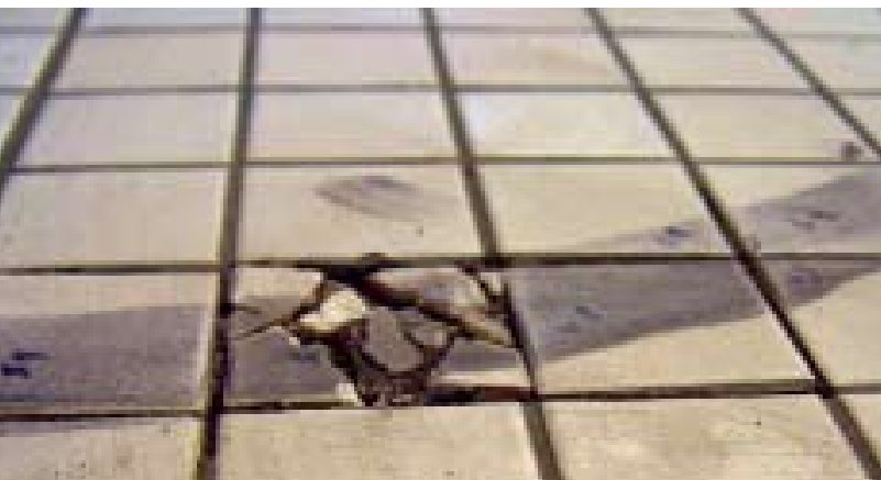
Below: The smaller the tile size, the larger the number of tiles and grout joints that come in contact with the wheel path. The image above shows an example of "broken tile" and "popped-up" grout joints.
